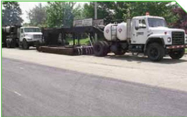
Two machines operating in tandem insure deep heating and softening of the aged pavement.
