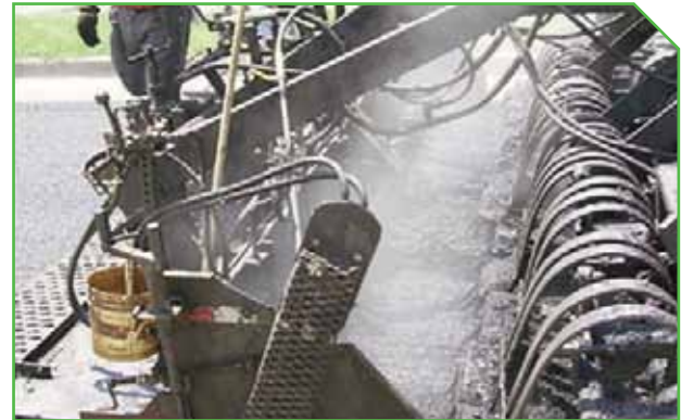
Multiple rows of spring loaded scarifiers penetrate the softened asphalt to the desired depth.
